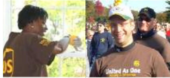
Shellie Olds-Johnson (CIM) paints a window for Habitat for Humanity in Roswell, GA.
